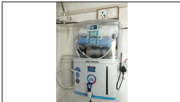
Fig. 116 A Kent RO water filtration system has been installed at our Garhaita base to insure abundant supply of clean drinking / cooking water, especially during intensely hot, pre-monsoon season in May-June. The unit is capable of filling 30 litre bottles quickly, so that fresh water is always available.
