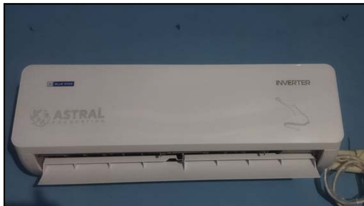
Fig. 114 A mini-split air conditioner was installed in the computer room at the Garhaita base, providing a climate control facility for operating electronics and for storing photographic and imaging gear during the monsoon. Unit allows both cooling and heating, and can be operated with assistance of generator when power is not available.
